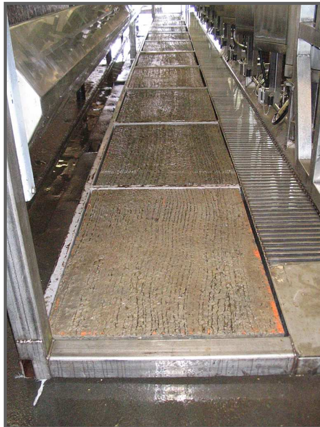
Ready-to-go cow platform one hour after parlor had been placed. Slabs will be replaced later on with poured concrete
