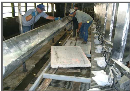
Each slab was cut a week ahead of time, numbered and cross referenced to its designated place.
