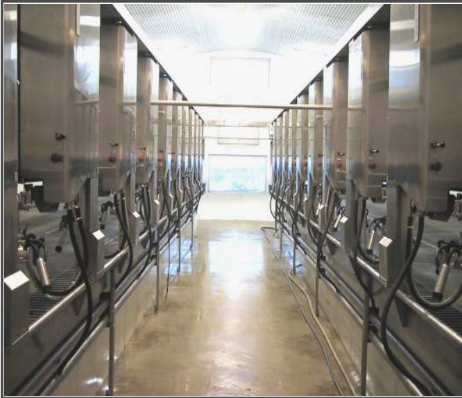
Dbl. 10 All-Stainless ProTime I HerringBone. Originally installed on a large dairy in Florida in 1989, milking 3,000 cows 3x.
